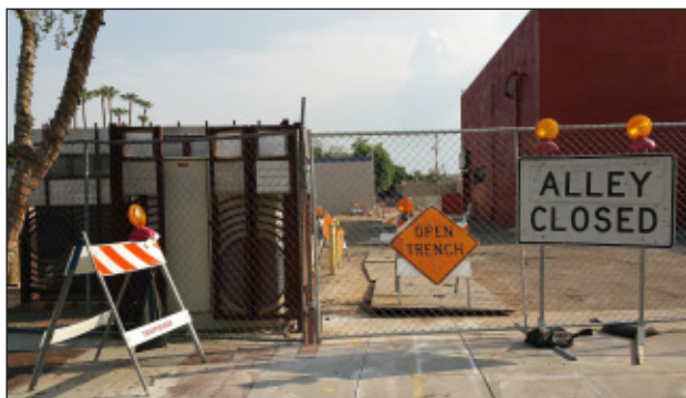
Fencing has been installed around the alley construction work area. The alley runs north and south, connecting Glenn Drive with Glendale Avenue between 57th Drive and 57th Avenue. During construction, there will be no public or business access to the alley to keep people safe and the project undisturbed. [Ed Sharpe/Glendale Daily Planet]
